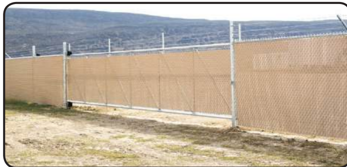
The entrance to the equipment yard has a large sliding gate to allow easy access for the Tribes' heavy equipment and other machinery. (Photos courtesy PrivacyLink®)
