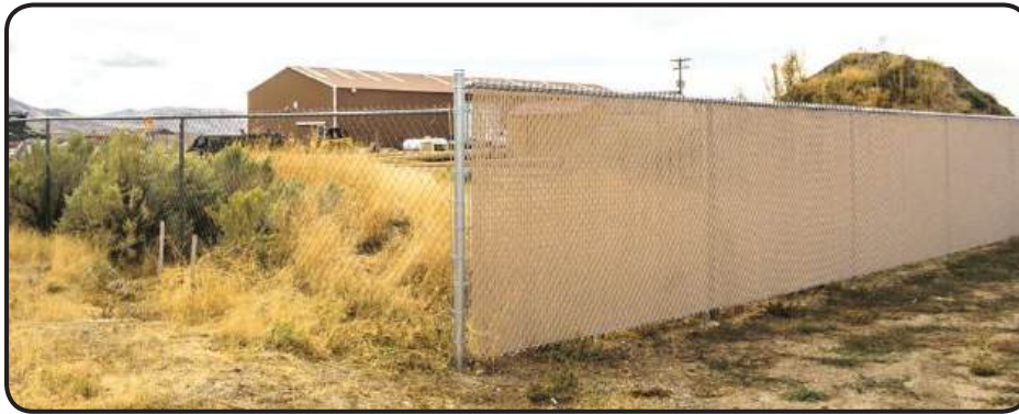
The new Noodle Link fence by PrivacyLink installed next to a section of the old fence at the maintenance yard shows the night-and-day difference the privacy slats made.
